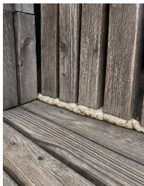
Obstruction of the ventilation cavity by foam, tape or unprotected insulation.
