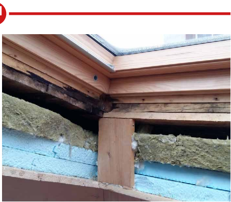
Window side detail: discontinuous insulation and irregular structural connections between timber, insulation and substrate, with a risk of air and water ingress and reduced thermal performance.
