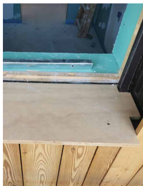
Details that do not drain retain water, such as window sills and horizontal joints.
