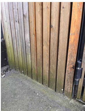
Discontinuous air inlets, with insufficient or interrupted inlet and outlet openings, for example at doors and windows, corners and chimneys.
