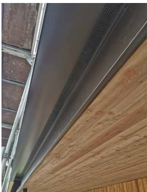
Continuous ventilation openings, free from debris or residue.
