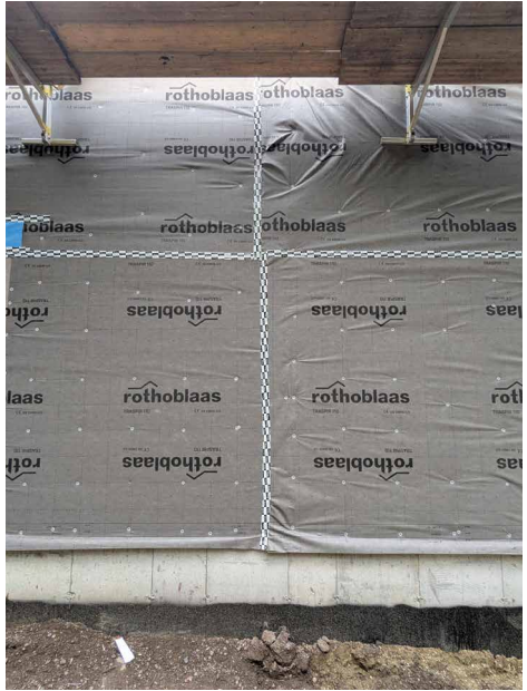
Aligned vertical joints create a preferential path for water ingress. Failure to tape ends and fastener penetrations.
