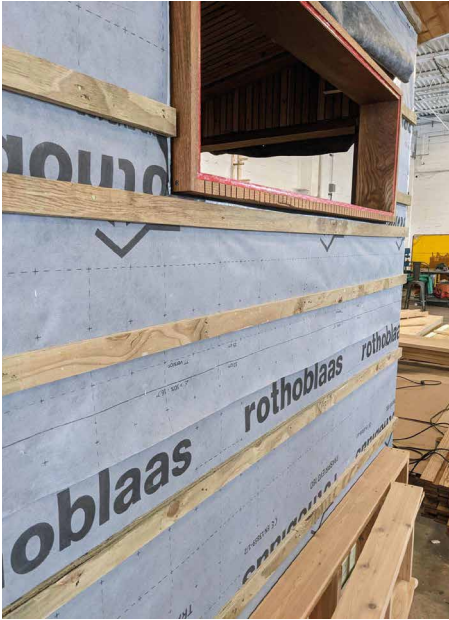
Membrane not taped with no nail sealing provided.
